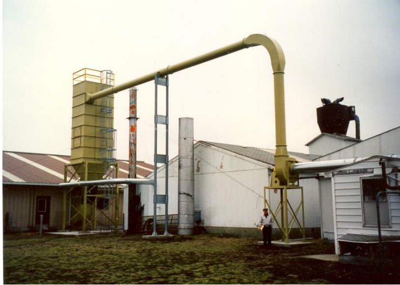
A sophisticated sawdust collection system, powered by a diesel engine, services an Amish carpentry shop.
